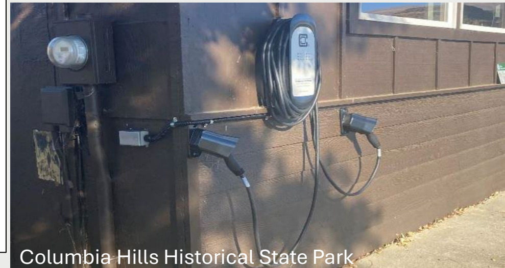
Example of Tier 1 fleet EV charging hub
