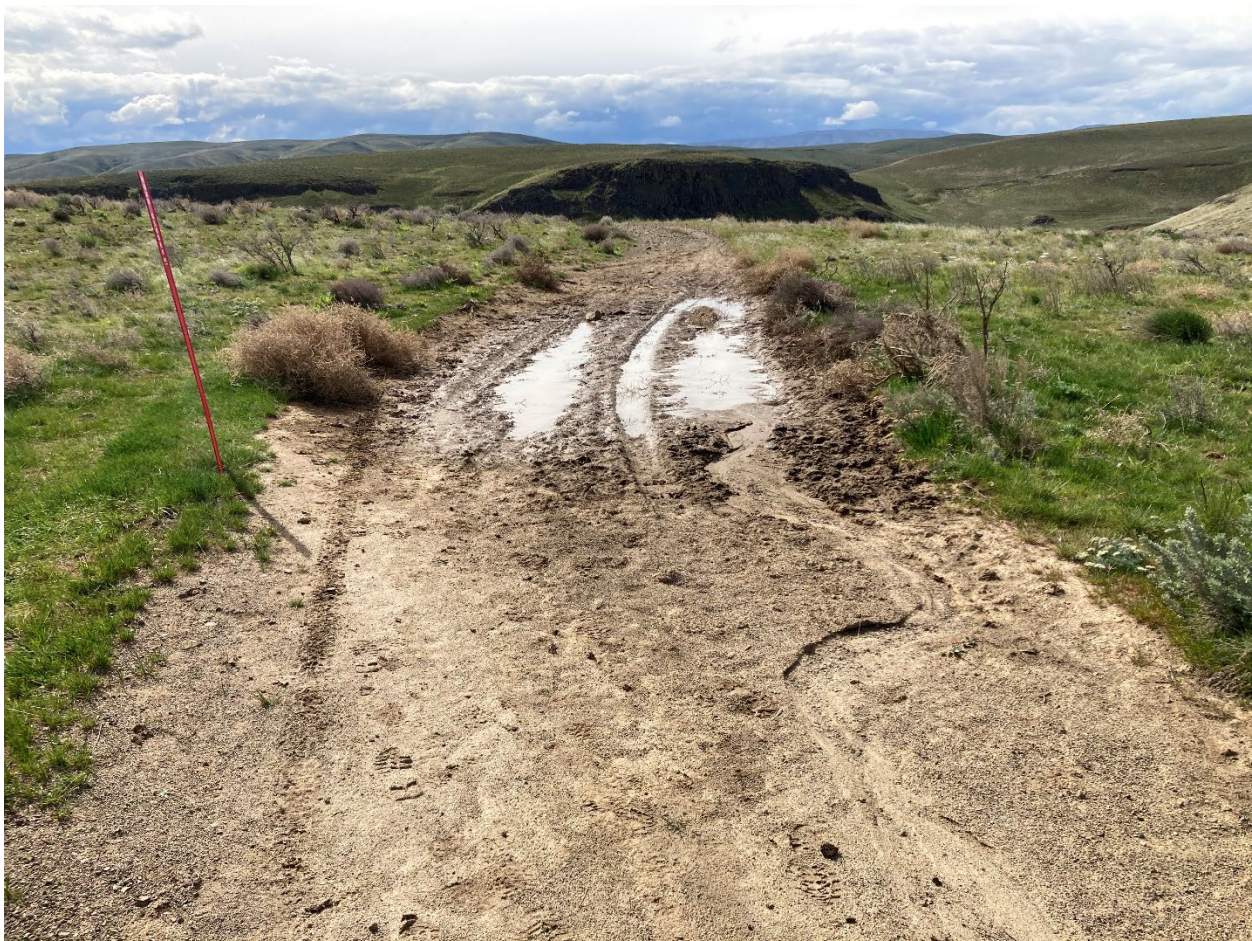
Photo 3. Sandy silt portion of Recreation Drive Trail with a puddle in the low spot. View is toward the south.
